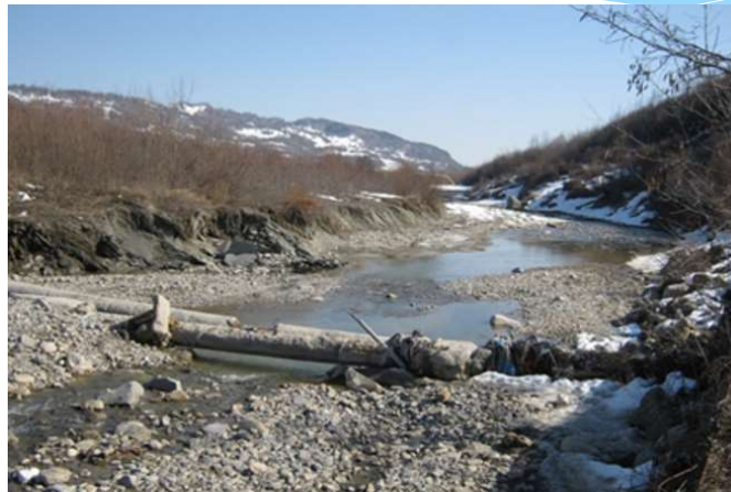
The D-erosion area- water pipes laying under the gravel bed may currently be seen at the water surface.
