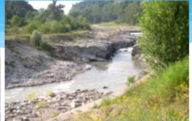
The E-erosion area- near Breaza town-Sărăcilă Valley. In August, 2006, the road was damaged by lateral erosion.
